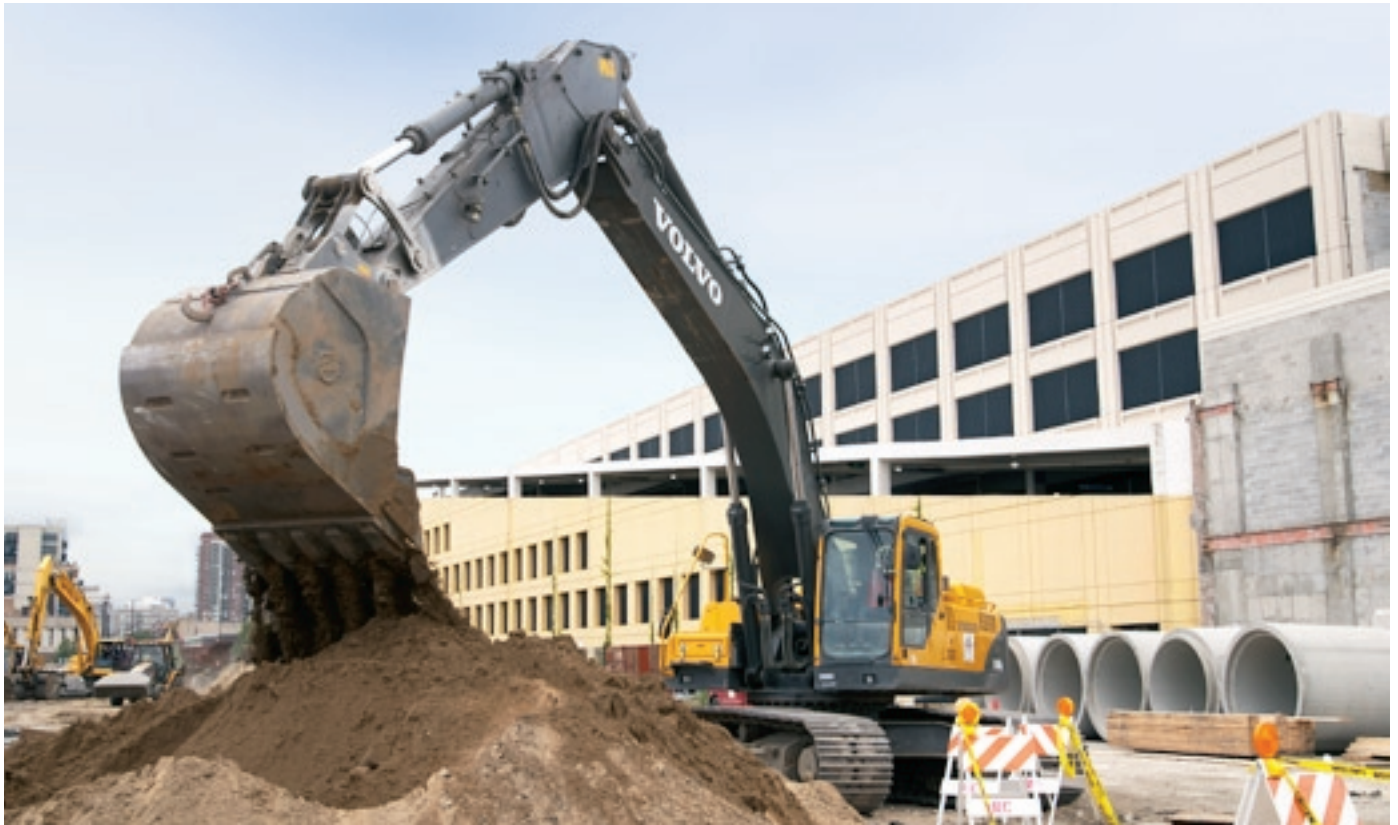
The storm drainage system that will link to the deep tunnel includes pump stations that will prevent backflow problems.
