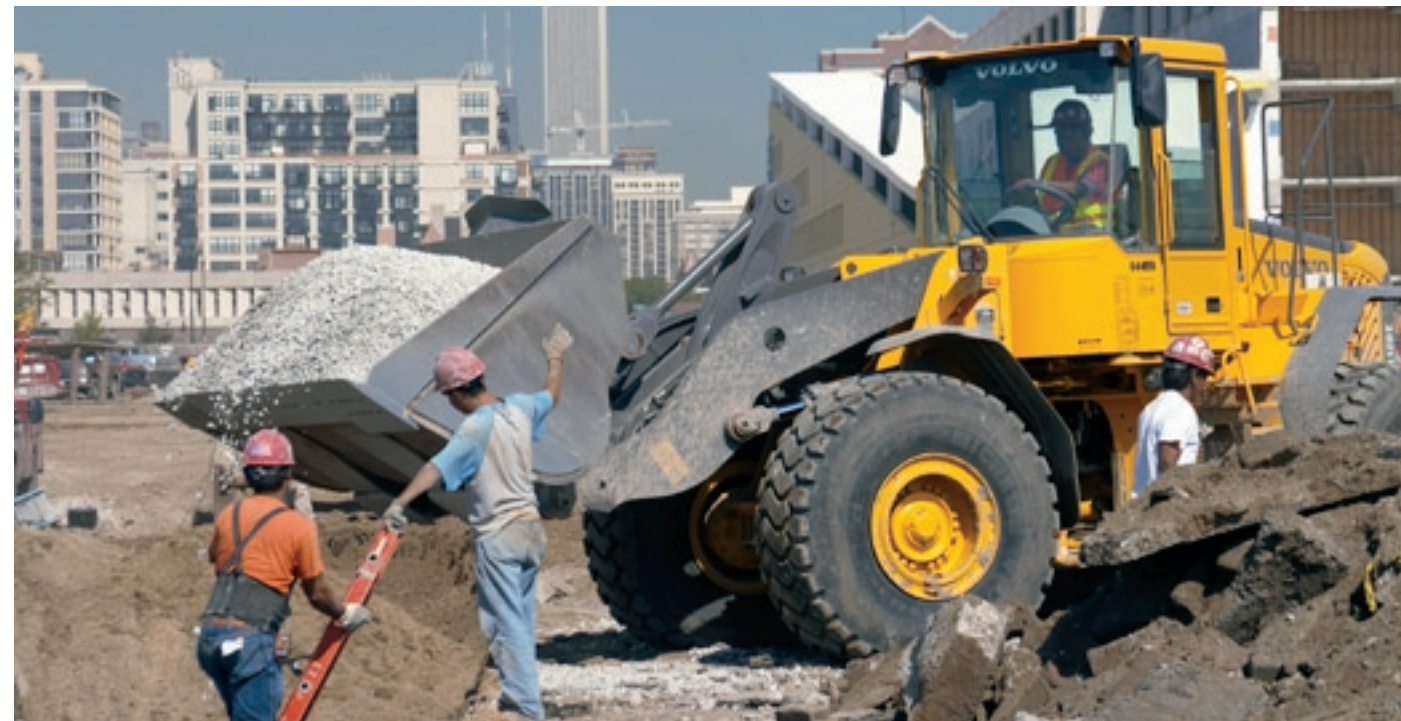
Reliable Contracting & Equipment Co. installed site utilities, including storm drainage running to the deep tunnel.
